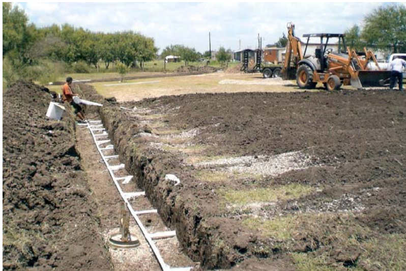
Septic system installed in Nueces County through the SEP program
